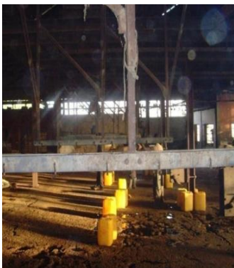
Fig. 7c: Hang rail in Sokoto abattoir vandalised (Lawan, Raji... et al. , 2013)
