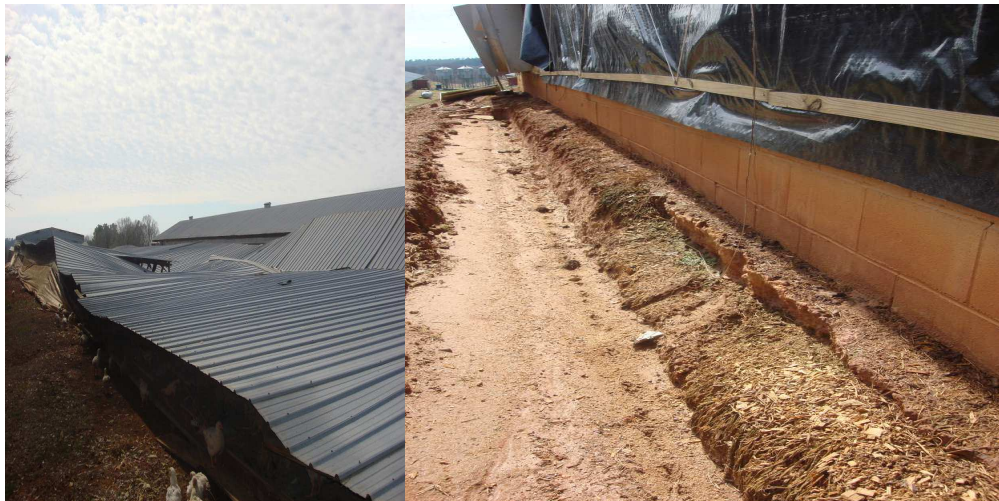
Figure 22. Poultry House Structural Failure Analysis
