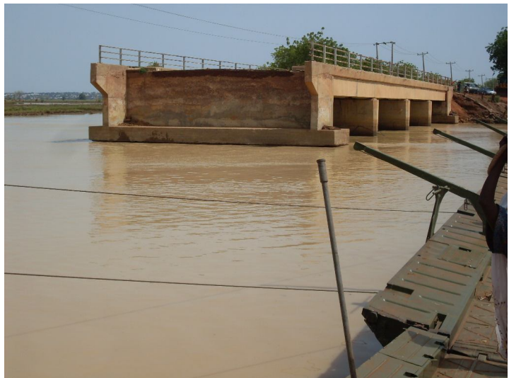
The access bridge on campus partly washed away by the devastating flood
